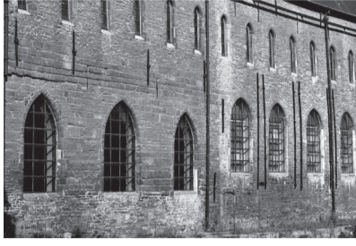
2. Pand monastery Intersection Predikherenlei and Hoornstraat, at the bridge over the Lys
